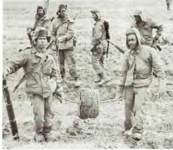
ENGINEERS AT WORK — Men of the 77th Cmbt. Engr. Bn. build a barbed wire fence below a Communist-held hill along the Han River, near Songnimong, Korea.
