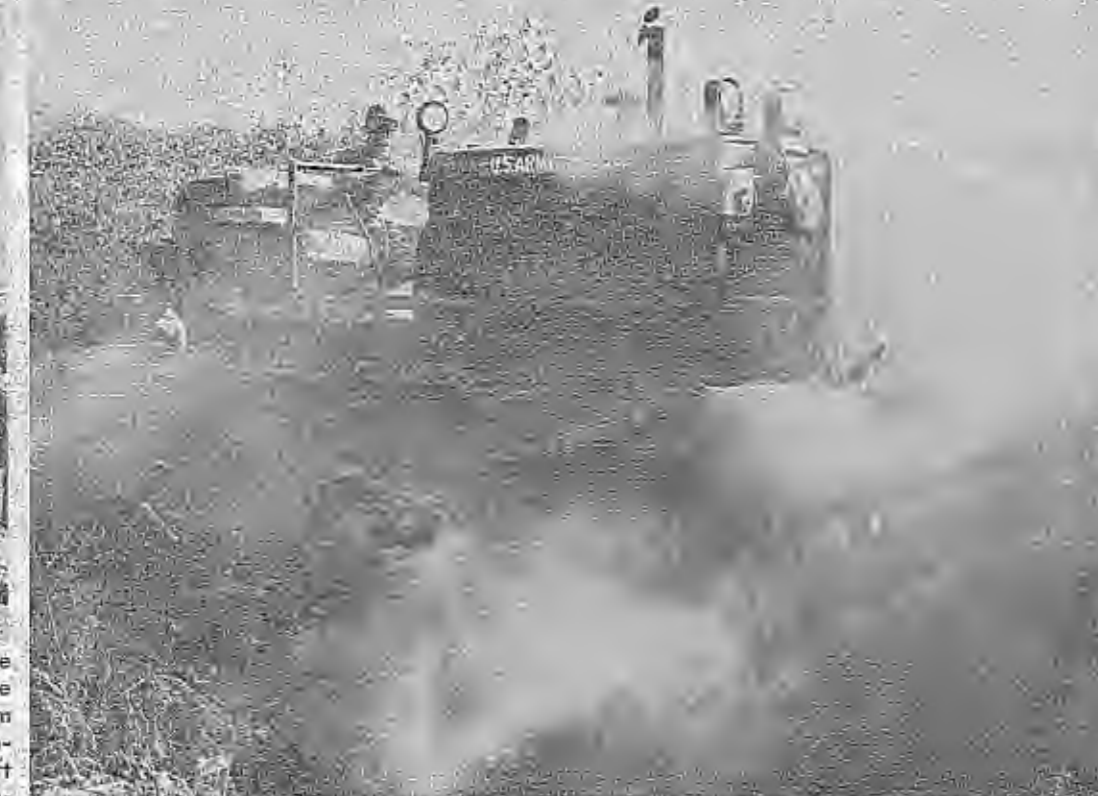
DUSTY WORK - Members of Co. C, 65th Eng. Bn., were hard at work pushing Bobcat Trail a little further into the impact area during their month at PTA. Sp4 Larry Bisling was one of the bulldozer operators.
