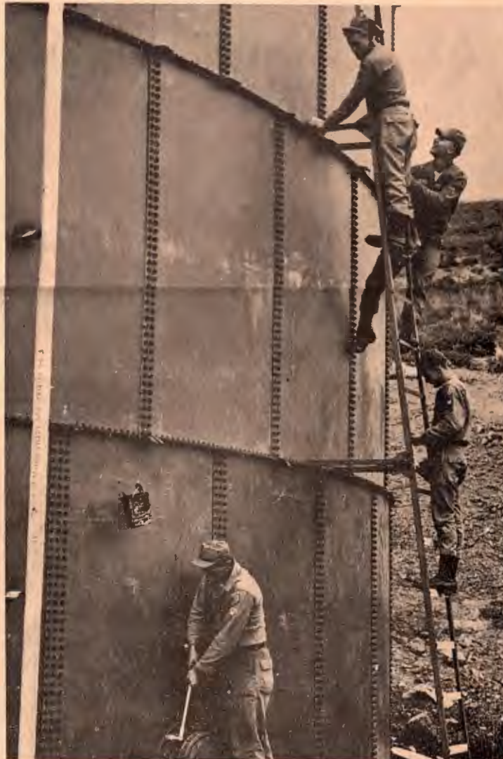
NEW TANK - Members of Co. B, 65th Engr. Bn., make final checks on the 420,000 gallon water tank they completed during their stay at PTA.
